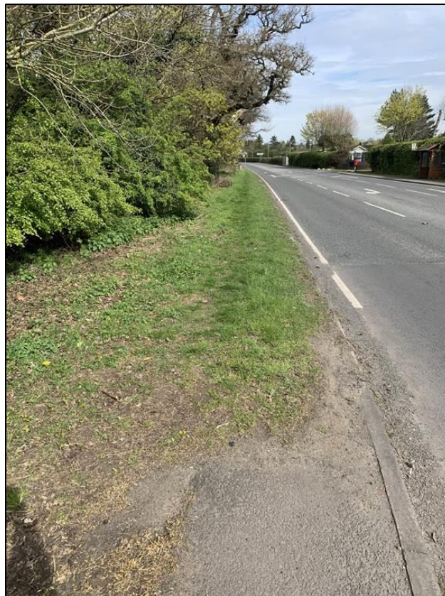
Worn verge where pedestrians are accessing the bus stop
