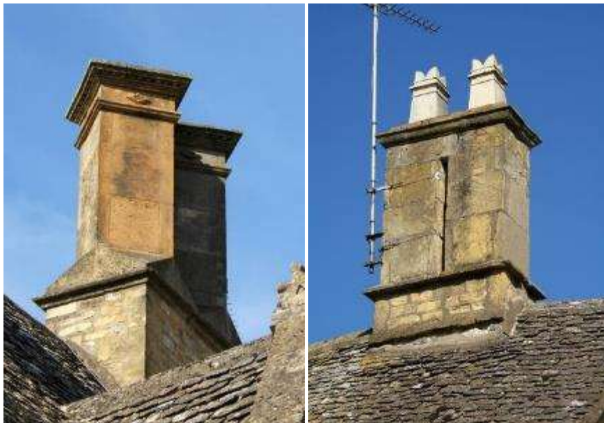
A double chimney in ashlar stone in Broadway (left) and with square pots (right)
