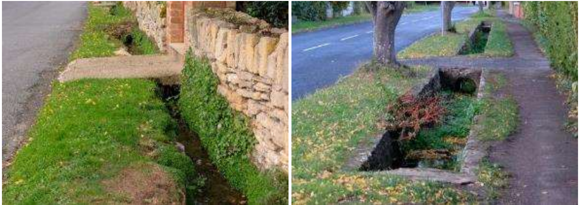
Open drainage ditches in Kemerton (left) and Elmley Castle (right) not only add character to streets but also provide a model for swales as part of a sustainable drainage strategy
