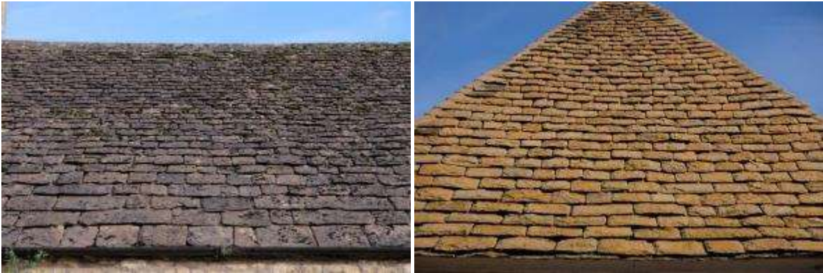
A traditional stone slate roof in the Cotswolds, the slates increasing in size down the roof (left). The colour of the stone slate can be quite orange when new (right), but it darkens as it ages and weathers.
