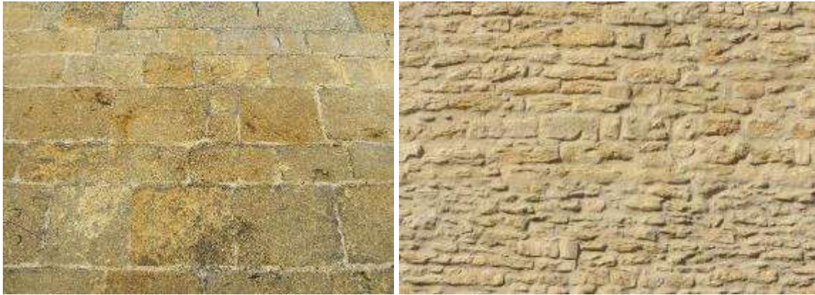
In dressed stone walls (left), the stones are squared off to give greater uniformity and a buttered stone wall laid in a thick bed of mortar (right)
