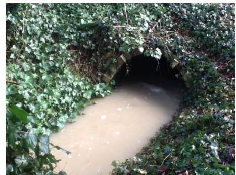
Entrance to the old culvert which cannot cope with extreme rainfall
